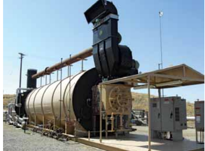
KERN COUNTY OIL FIELDS QLN-II™ INSTALLATION
