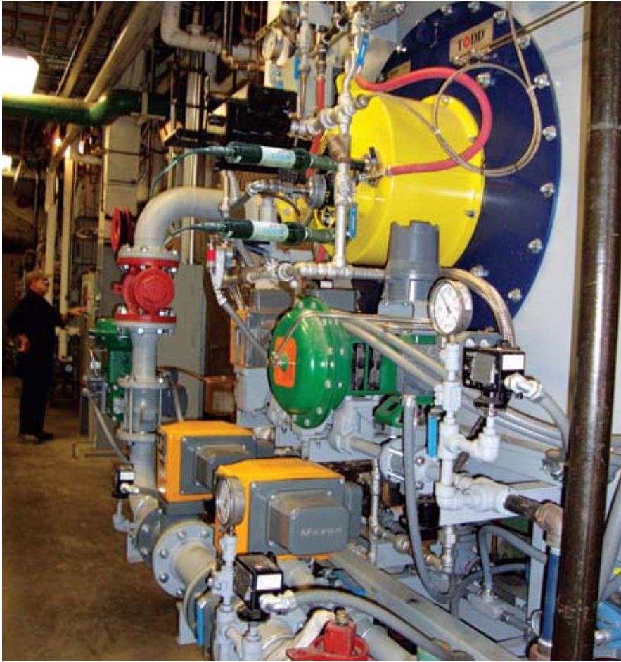
FIGURE 1 WATERTUBE BOILER INSTALLATION
