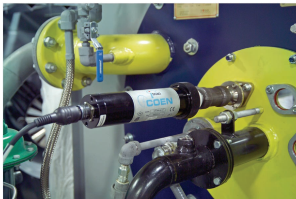
Figure 4. iScan mounted on the back of a burner.
