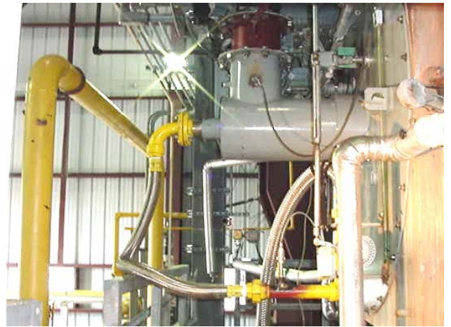
Delta-NOx ULN Installation at Calpine
