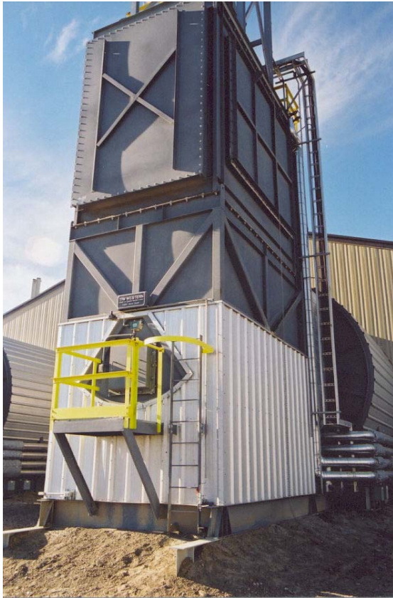
Back End View of Steam Flood Unit
