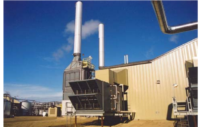
2 of 4 Steam Flood Units in Alberta
