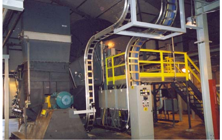
Coen QLN 4.8 with FD Fan and Controls
