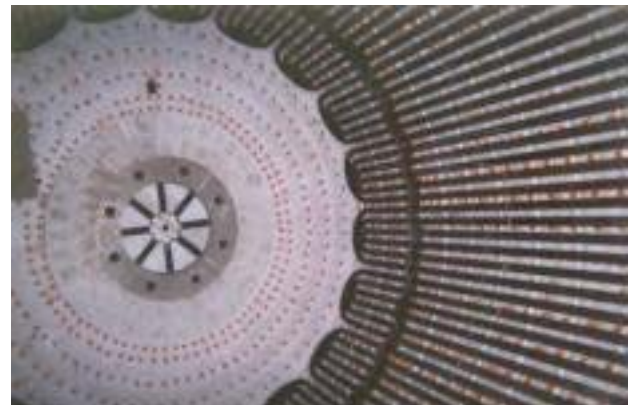
Coen QLN 4.8 Burner, Inside Furnace
