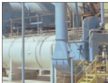
Refractory Lined Furnaces
