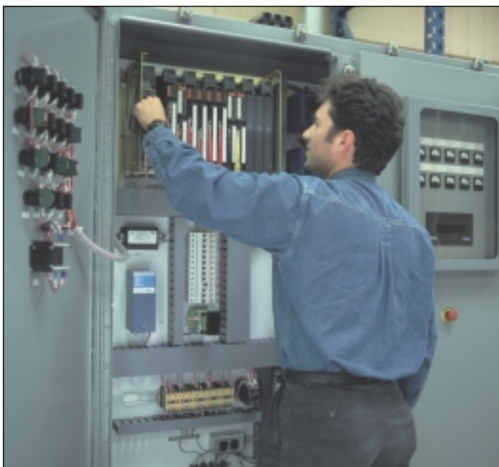
Control Panels & Piping Systems
