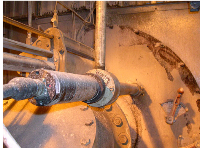
iScan Installed at Burner Front
