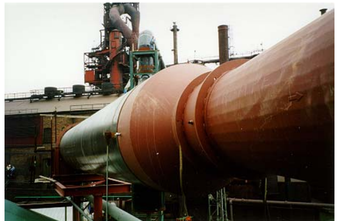
Fig. 2 Large 72" BFG supply line to boiler house
