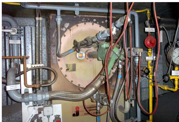
Burner Front at GMK Power Plant
