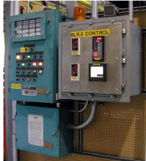
Simple BMS & Control Panel
